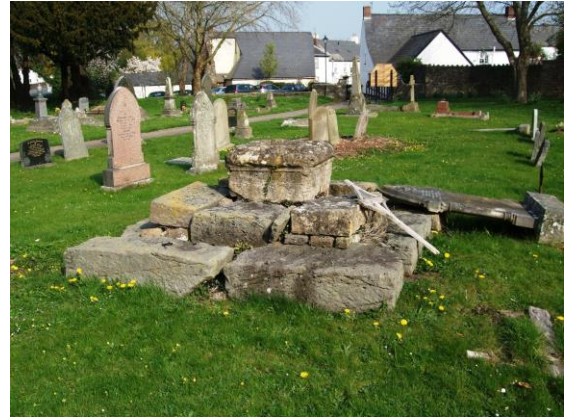
Fig.31 The medieval cross base in a poor state of repair
