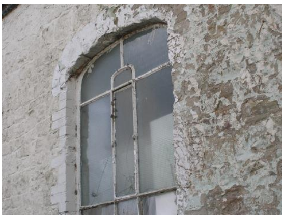
Fig.78 Former Chapel, West End. A detail of the unusual and elegant metal window frames.
